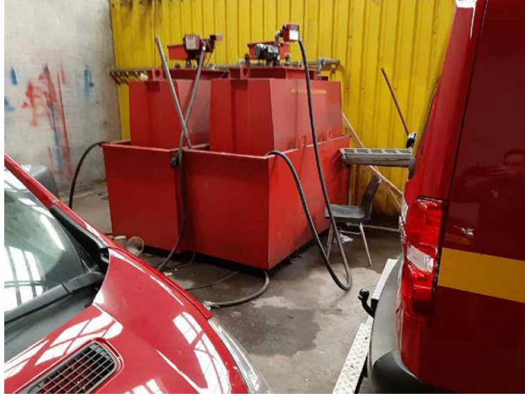
Dieseltanks in bak
