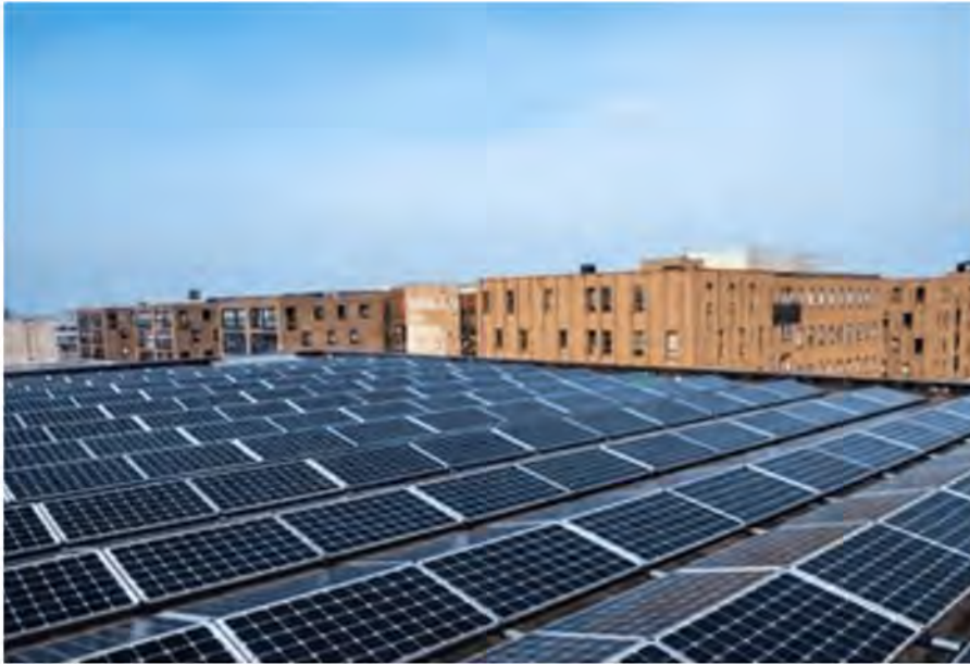
PV-panelen IJburg college
