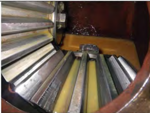
Detailfoto 7: Schade tandwiel inkomende as HTK 4
