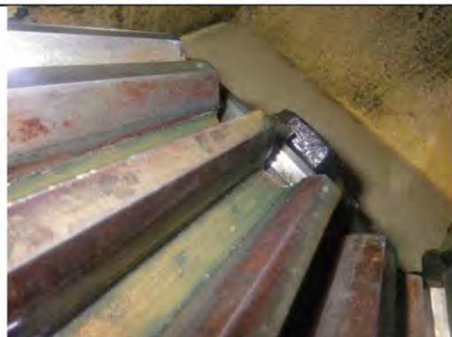
Detailfoto 9: Schade tandwiel inkomende as HTK 1
